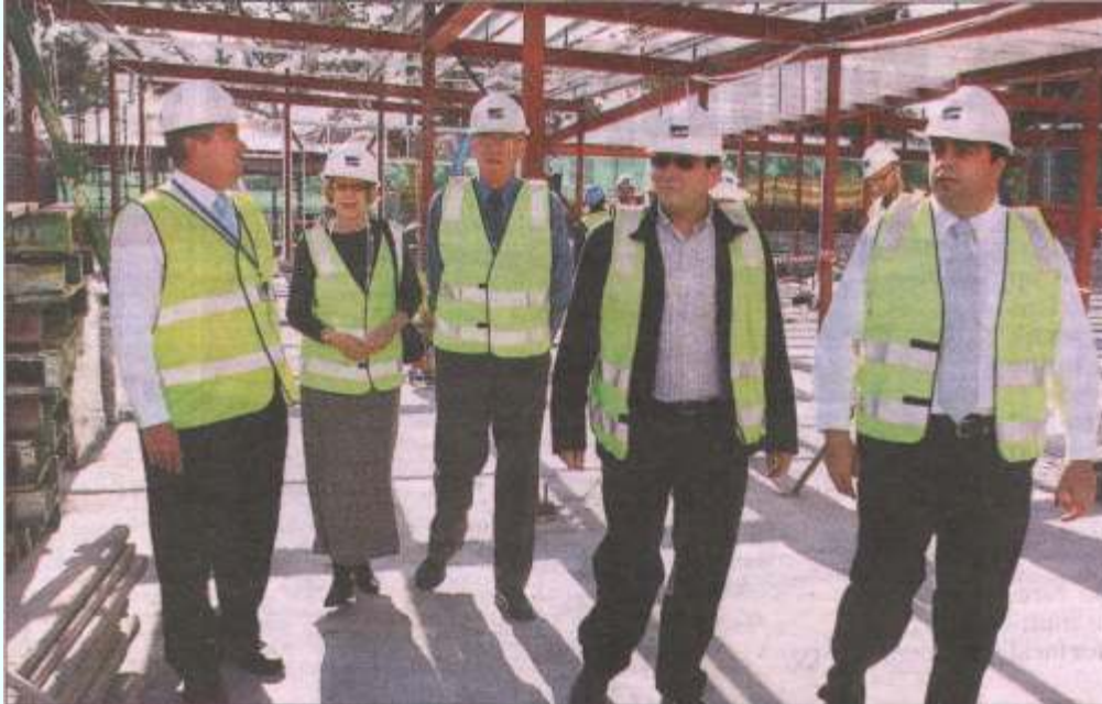
Building up: Karitane executive manager Robert Mills, chairperson Professor Bryanne Barnett, vice-chairman Michael Coffey and project manager Nigel Jones show Fairfield MP Joe Tripodi over the site. "The new capital works are being funded from Karitane's trust funds and a NSW Health grant of $1 million," Mr Tripodi said . Picture: Helen Nezdropa
